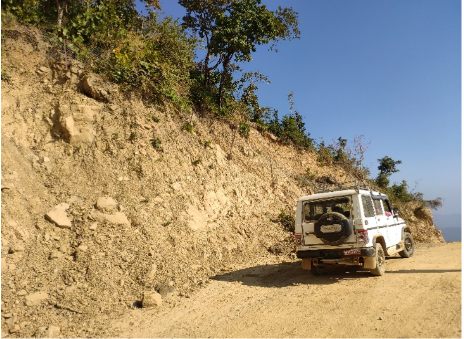
Figure 19: Shallow landslide below Devikot temple due to new road cut
