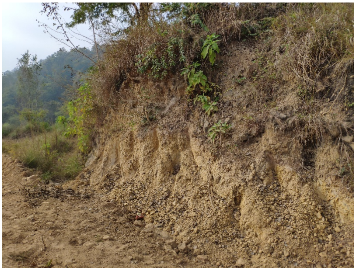
Figure 9: Mudstone almost weathered show soil like nature
