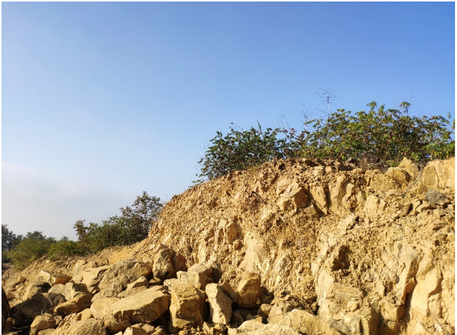
Figure 18: Wedge failure and rock fall in Middle Siwaliks
